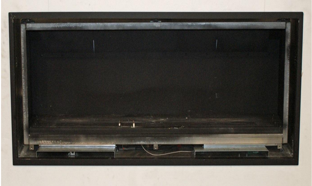
Empty Fire box
